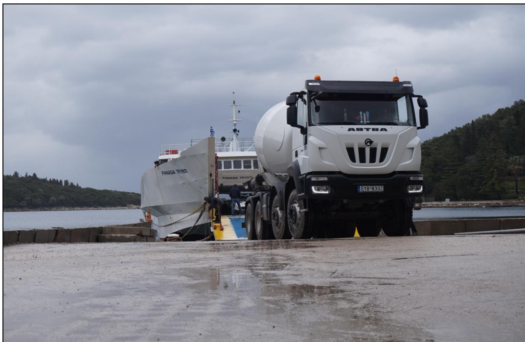
Figure 2.1-12. Transport of materials that are used in the project in quantities that require more than five trucks per day, are carried outside of the island according to a material transport plan.
