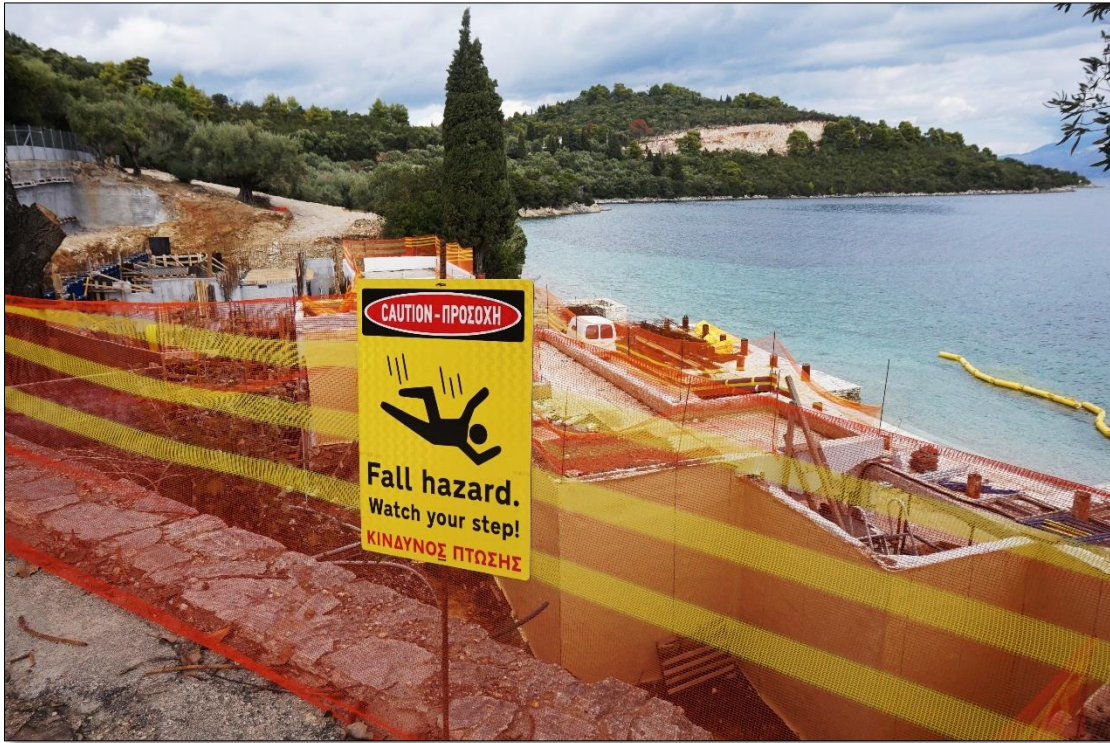
Figure 2.1-2: Warning signs and protective net in Local construction site near the sea.
