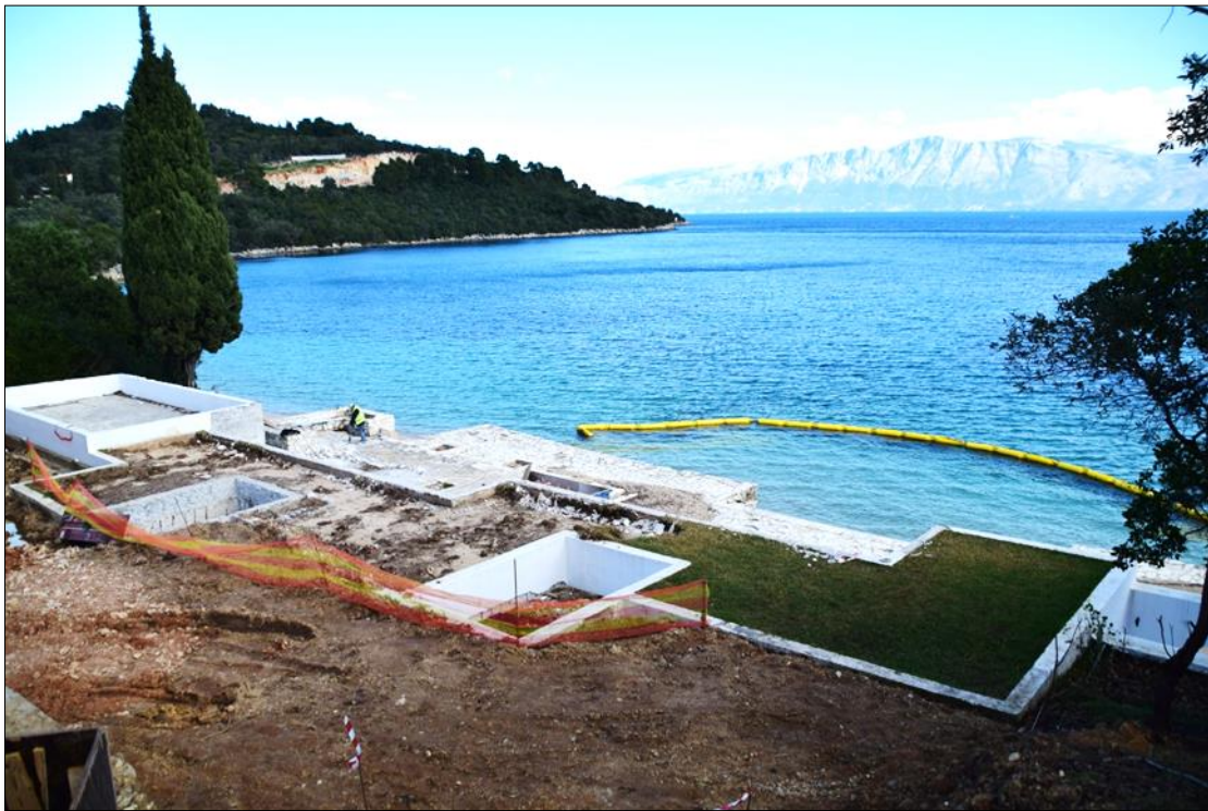
Figure 2.3-1: Works in progress at Local construction site near the sea. Silt curtain in place for protection.
