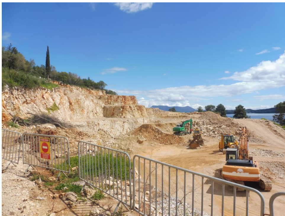
Figure 2.1.3-1. Marking of the project's working spaces with suitable fences and warning signs.
